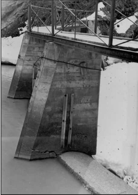
Figure 13. Catwalk installed on diversion dam in 1933 at request of FPC. Courtesy of National Archives, AK Region, APA Box 42.
