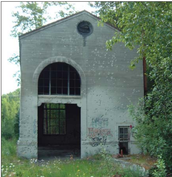
Figure 44. Front view of powerhouse as it appears today. Note that the left lean-to addition (switchroom) is no longer present. Date removed unknown. Photo by R. Sackett, June 2001.
