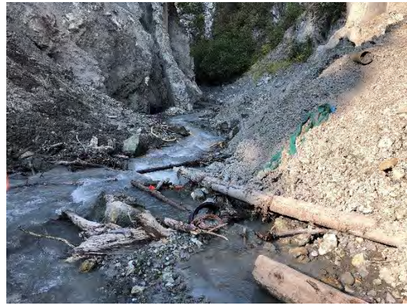
Figure 28: Miscellaneous construction debris
