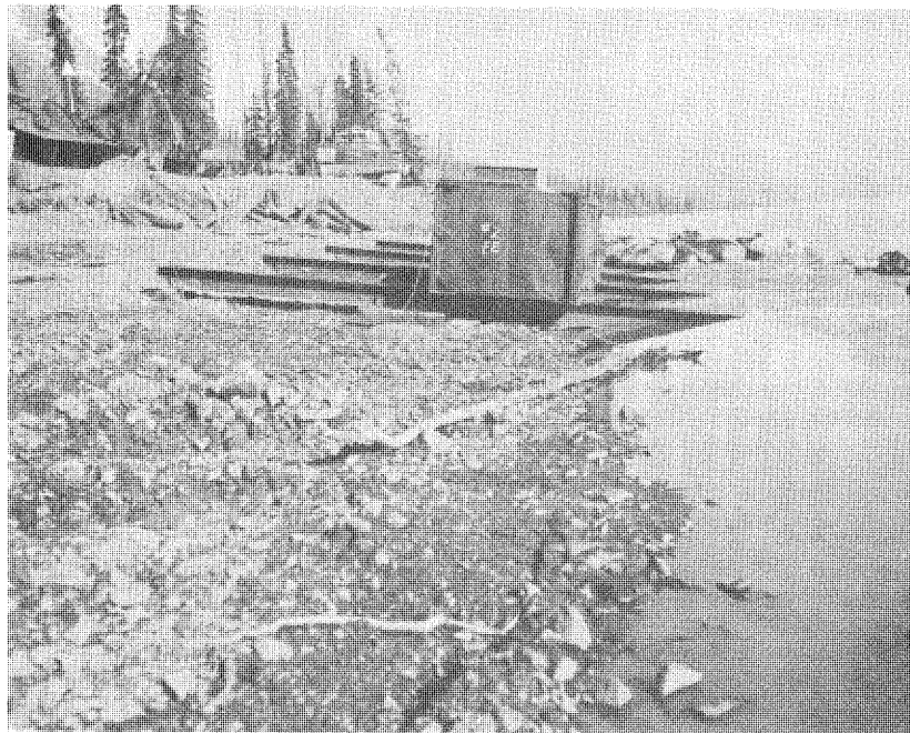
Figure 104. --View of assembly area for dredge at Eklutna Lake showing one steel pontoon and steel skids on which assembled dredge will slide into lake. P783-908-788, May 2, 1952.
