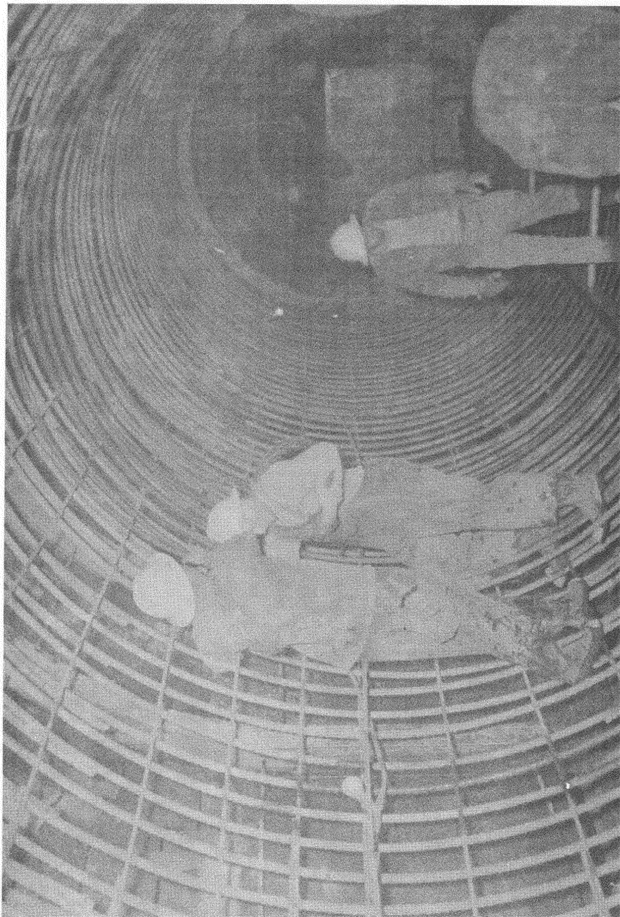
Figure 30. --Reinforcement steel in tunnel section at station 20+50. Steel forms are in background. P783-903-926, June 25, 1952.
