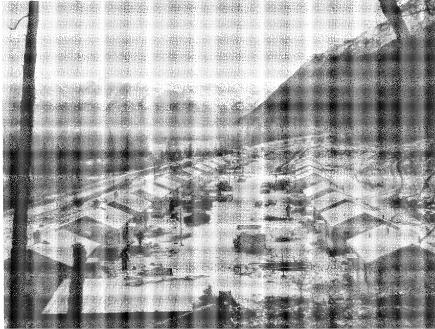
Figure 102. --Temporary and permanent houses under construction at Eklutna Government camp. P783-908-459. November 27, 1951.
