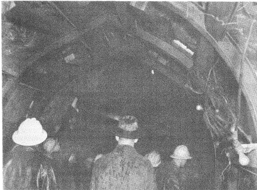
Figure 113. --Contractor's men erecting steel support in main tunnel at location of a vertical fault, near station 242+45. Temporary timber lagging is shown inserted in roof of tunnel to protect workmen raising supporting steel. P783-908-752, April 7, 1952.
