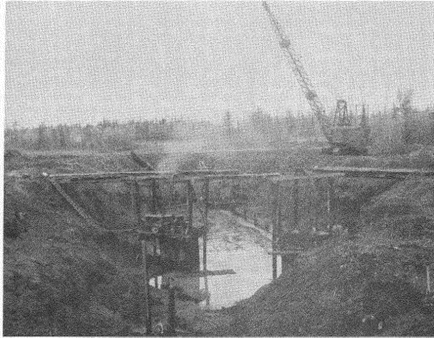
Figure 123.--General view of powerhouse and tailrace excavation showing pumps necessary to unwater foundation excavation. Shown are two 10-inch and three 6-inch pumps. P783-908-1084, September 19, 1952.
