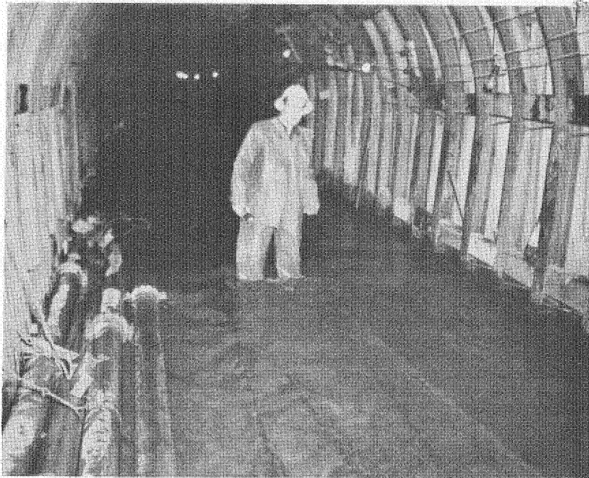
Figure 112. --Water flowing through tunnel from fault at station 208+70. P783-908-1163, November 15, 1952.
