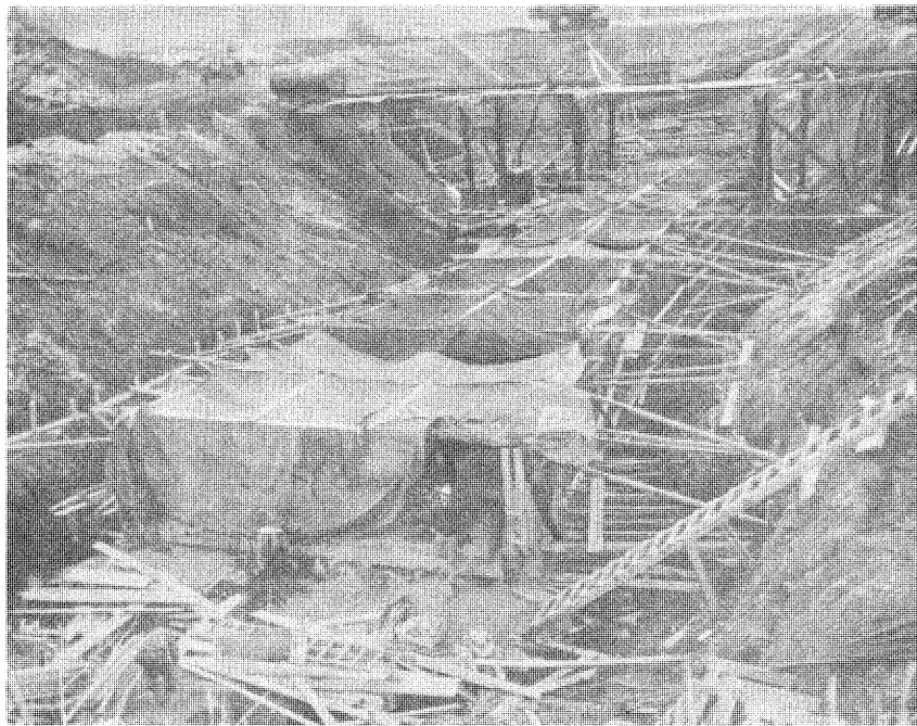
Figure 133. --Construction view of tailrace conduit, showing method of protecting newly placed concrete from freezing temperatures. P783-908-1118, October 18, 1952.
