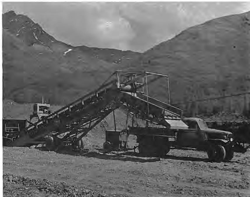
Figure 58. --Gravel processing plant, or separator, located in borrow area H. P783-908 C&R-122A, June 10, 1965.
