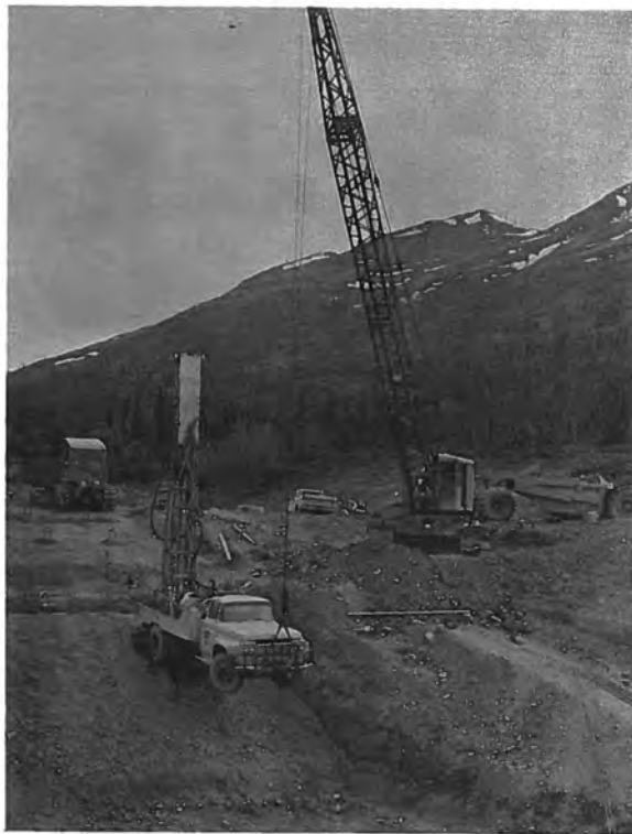
Figure 61. --Drill rig supported by motor crane while drilling holes for anchor bars on the spillway. P783-908 C&R-142NA, June 25, 1965.
