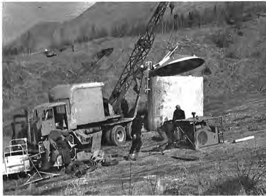
Figure 35. --Bureau and contractor personnel lowering diving gear into headgate shaft in preparation for investigation of conditions in and around the headgate seat prior to unwatering tunnel. P783-906-2319, May 9, 1964.
