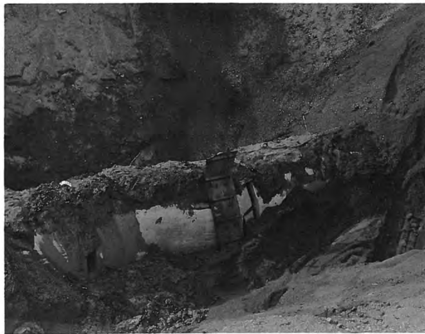
Figure 50. --Two damaged joints on the existing 9-foot-diameter precast concrete conduit. P783-908 C&R-27A, March 21, 1965.
