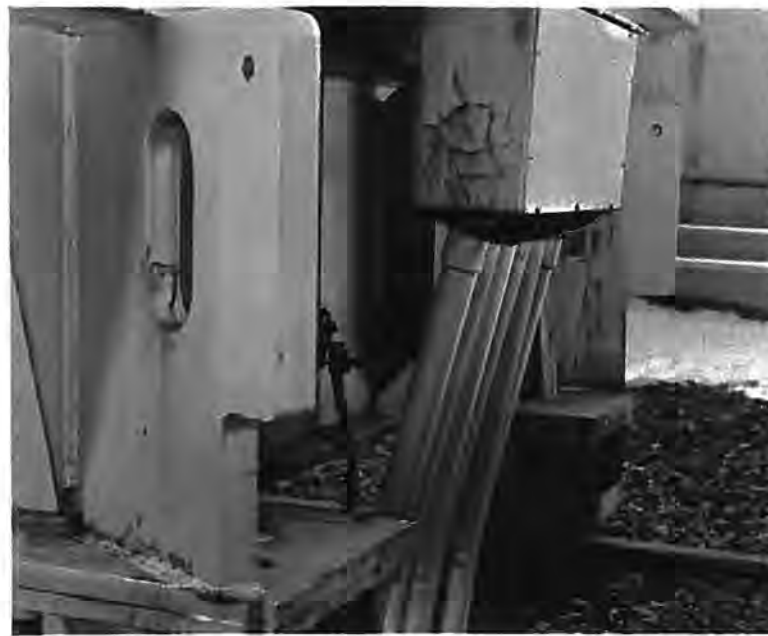
Figure 33. --View of 20,000-kv. -a. transformer conduit and terminal box showing damage caused by movement of the transformer during the earthquake. Rail stops, consisting of 1/4-inch by 1-inch-wide steel bars, were tack-welded to the rails. The welds broke and allowed the transformer to move on the rails. P783-906-2254NA, April 6, 1964.
