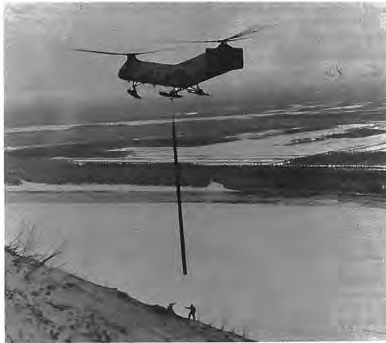
Figure 34. --View of helicopter assisting in reconstruction of 115-kilovolt transmission line. An Army helicopter crew cooperated with Bureau of Reclamation and Matanuska Electric Association line crews in rebuilding a section of the 115-kilovolt line which was swept away by a snowslide released during the earthquake. P783-906-2312, April 3, 1964.
