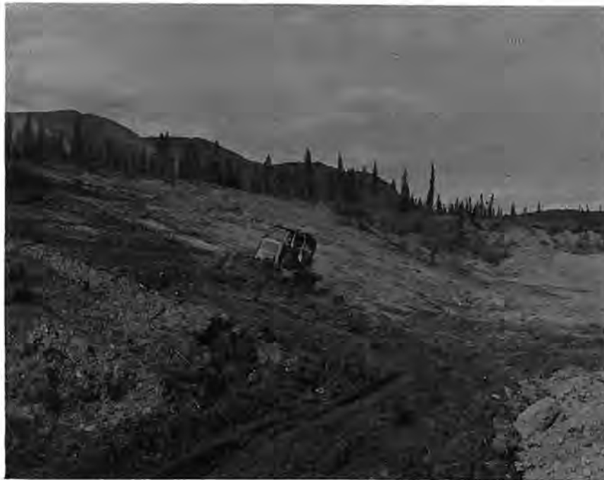
Figure 57. --Excavating operations on the left abutment of the new dam. P783-908 C&R-121A, June 10, 1965.
