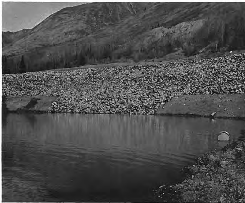
Figure 55. --Completed riprap in place on the backslope to the new intake structure. P783-908 C&R-83A, May 18, 1965.
