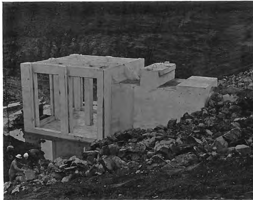
Figure 53. --New intake structure with concrete work completed and ready for installation of trashracks on the top, sides, and front. P783-908 C&R-65A, April 30, 1965.
