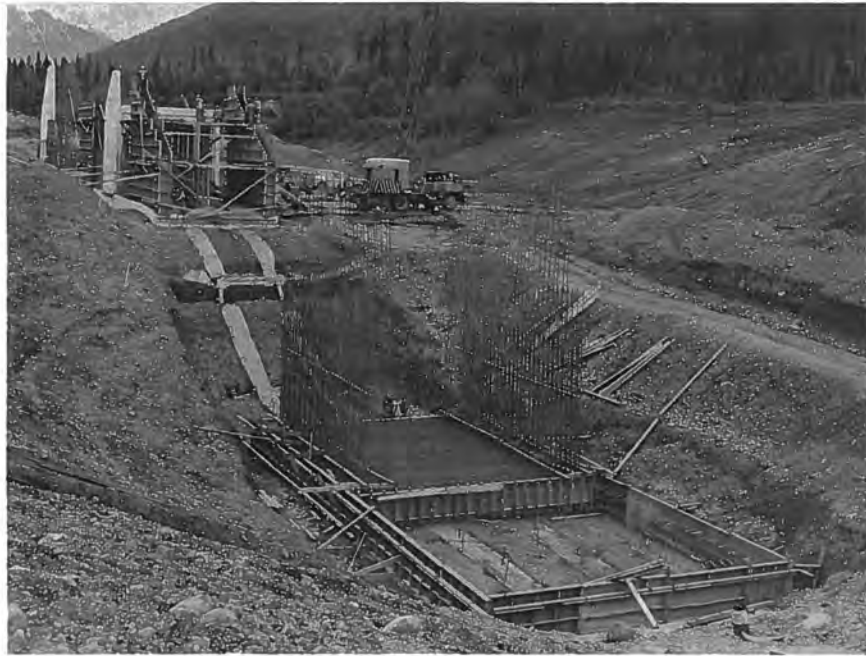
Figure 63. --Forming and steel reinforcement in the spillway stilling basin. P783-908 C&R-158NA, July 23, 1965.
