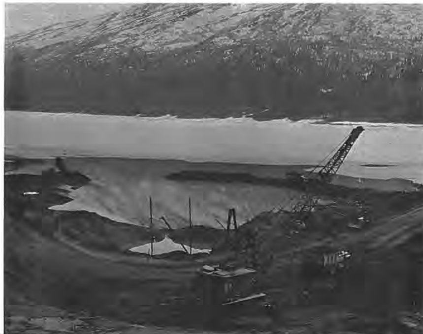
Figure 48. --General view of construction of cofferdam and excavation for the new intake structure. P783-908 C&R-7A, March 23, 1965.
