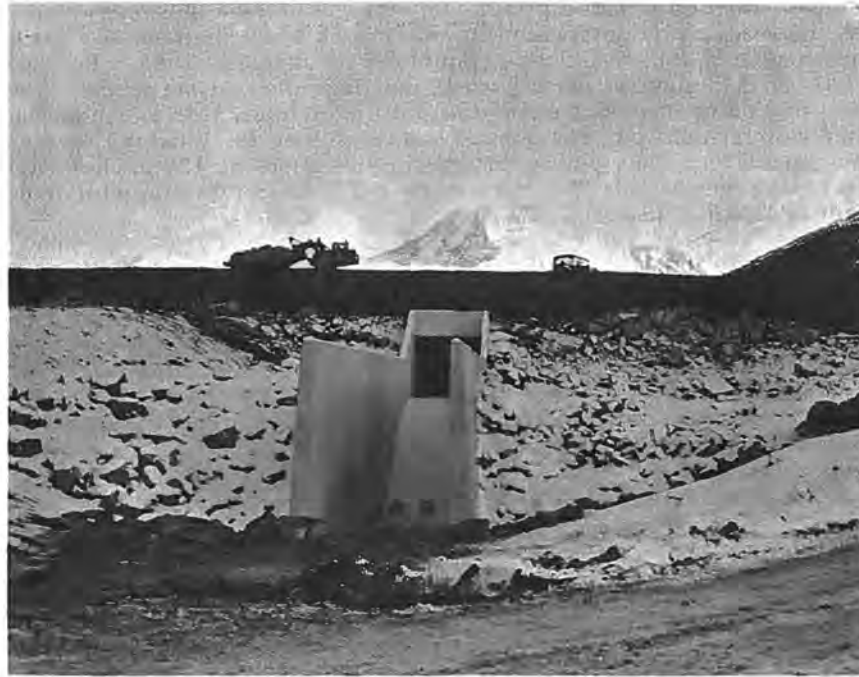
Figure 60. --View of the downstream face of the completed dam and spillway. P783-908 C&R-211NA, October 21, 1965.
