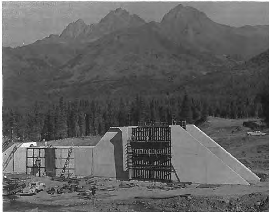
Figure 65. --Concrete placements on the inlet and conduit sections of the spillway nearing completion. P783-908 C&R-172NA, August 19, 1965.
