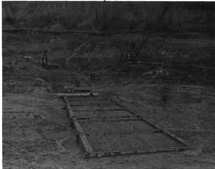
Figure 49. --View showing exposed top side (trashracked side) of original intake structure after removal of water. P783-908 C&R-17A, March 26, 1965.
