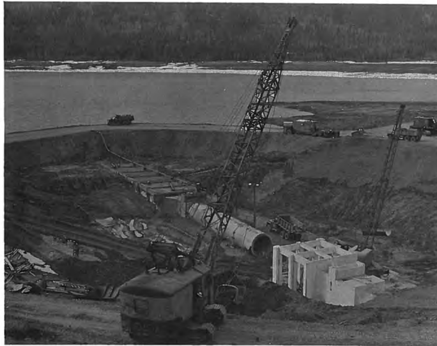
Figure 51. --General view of abandoned intake structure and conduit in the background and new intake structure nearing completion in the foreground. P783-908 C&R-54A, April 28, 1965.
