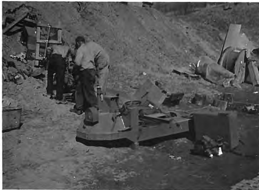
Figure 42. --View of diesel-powered 1-1/2-cubic-yard haul unit being dismantled prior to lowering it into the tunnel through the headgate shaft. P783-906-2343, June 1964.
