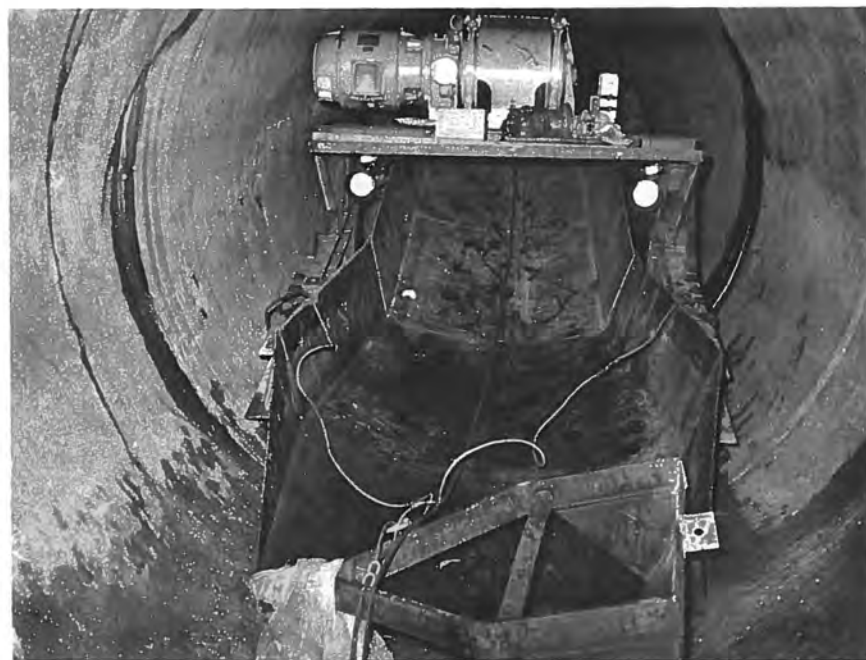
Figure 44. --View of loading chute and drag bucket of the 15-horsepower electric slusher unit used by the contractor to remove accumulated gravel from the pressure tunnel. P783-906-2349, June 1964.
