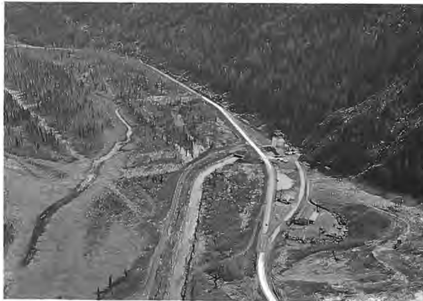
Figure 32. --General view of Eklutna Powerplant after the earthquake. Cracks up to 5 feet wide along the banks of the 2,000-foot tailrace channel are clearly visible below the powerplant. The cracks had the effect of squeezing in the sides of the channel. The channel was cleaned by means of both blasting and dragline operation. P783-D-44504A.
