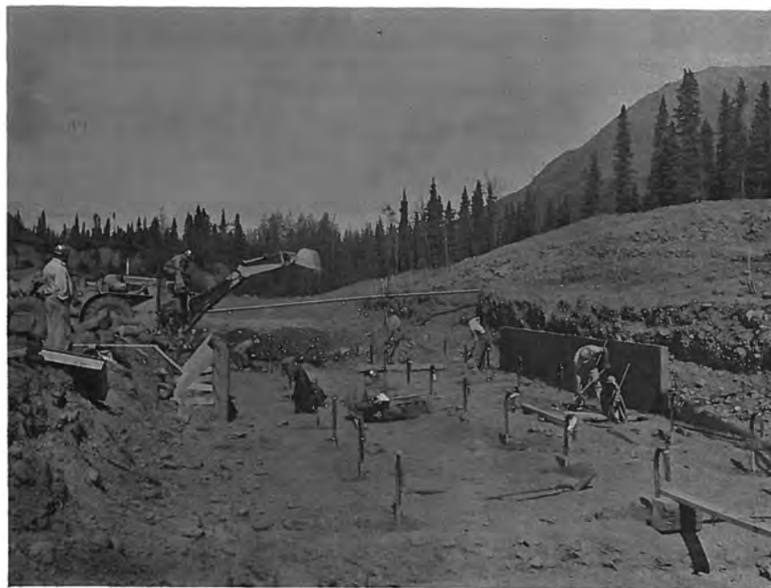
Figure 62. --Anchor bars in place on the spillway structure subgrade. P783-908 C&R-113A, June 10, 1965.
