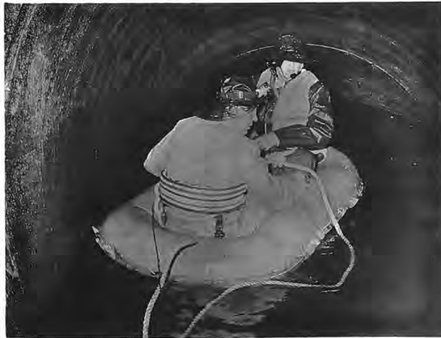
Figure 36. --A two-man rubber raft being used for internal inspection of the 863-foot-long penstock which slopes at an angle of 53^\circ with the horizontal. Descent of the raft was controlled by releasing water from the penstock drainlines. P783-906-2315, May 18, 1964.
