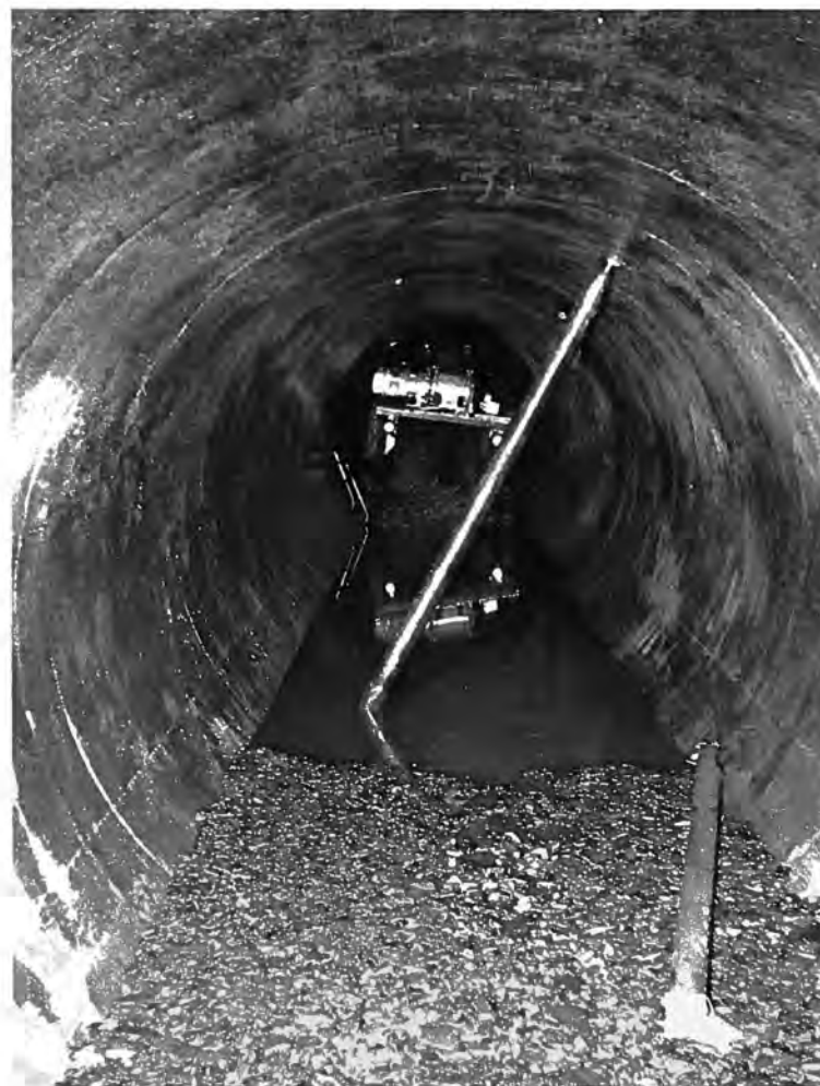
Figure 45. -- Accumulation of debris in pressure tunnel as a result of earthquake damage to pre-cast concrete intake conduit. Rock in foreground is typical of that deposited throughout 3-1/2 miles of the tunnel. View is looking upstream toward the loading end of the slusher unit. The drag bucket is being drawn toward the slusher from the gin pole in the center of the picture. P783-906-2351, June 1964.
