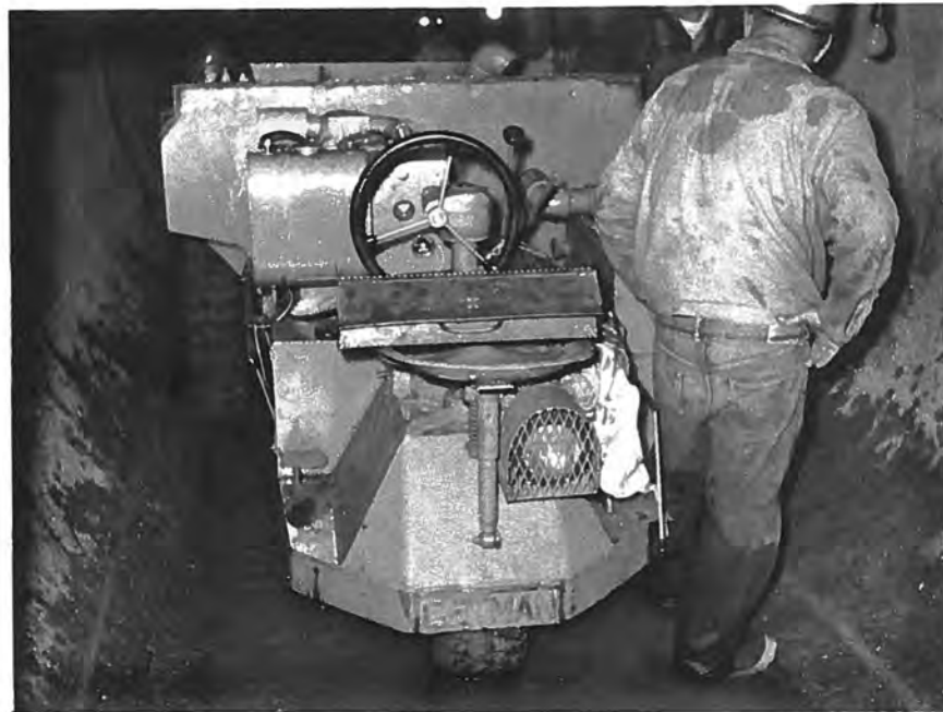
Figure 43. --View of the haul unit being reassembled in the 9-foot-diameter tunnel. P783-906-2344, June 1964.
