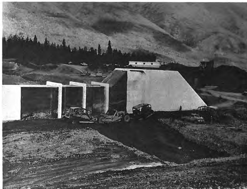
Figure 66. --Butyl-rubber covering in place on the conduit section of the spillway. P783-908 C&R-184A. September 2, 1965.
