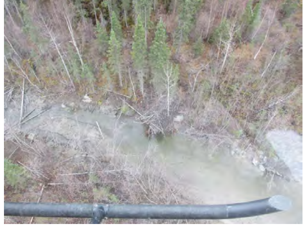
Figure A.2-14. Inactive Lodge-04 in the upper river colony. Beavers from this colony were trapped and removed by the Alaska Department of Fish and Game and the dam was removed with heavy machinery.
