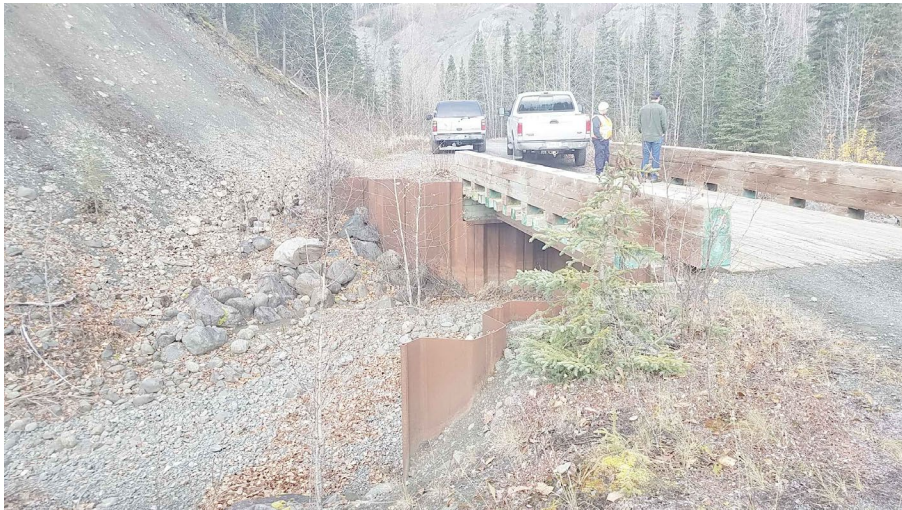
PROPOSED CROSSING BRIDGE EXAMPLE - LOOKING AT UPSTREAM SECTION OF BRIDGE FROM ROAD GRADE SCALE: NTS
