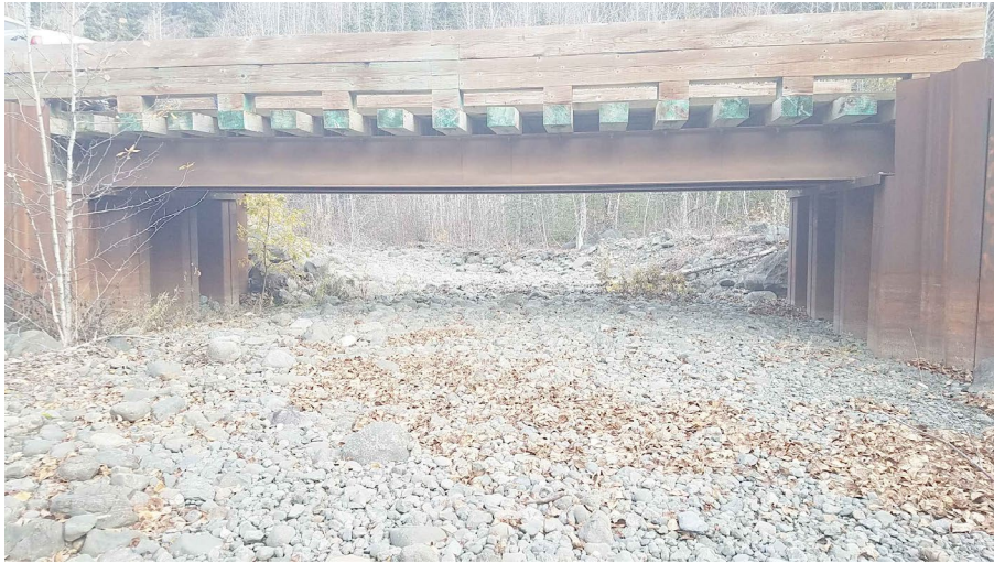
PROPOSED CROSSING BRIDGE EXAMPLE - SECTION VIEW FROM RIVER BED LOOKING DOWNSTREAM SCALE: NTS
