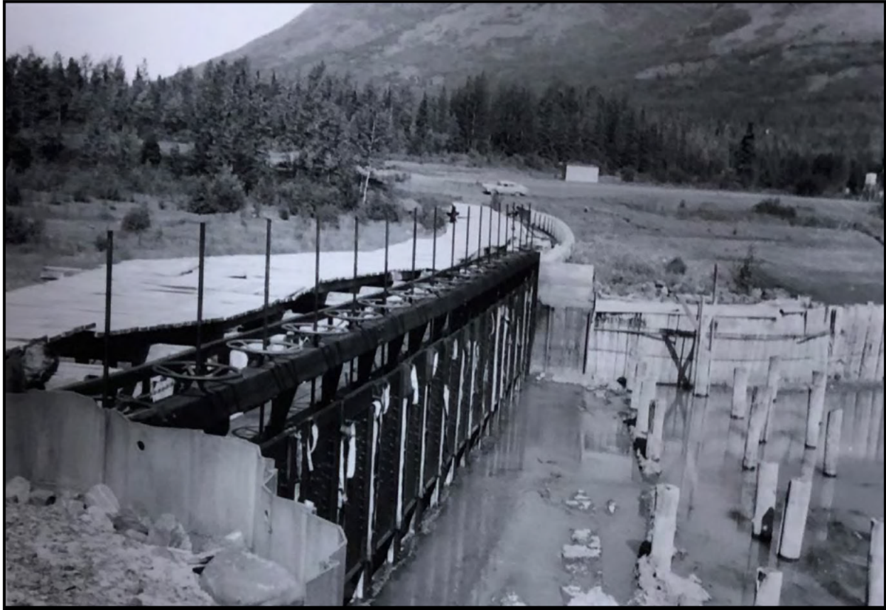
Figure 5.2-17. Photograph of the Eklutna Dam and Spillway following the 1964 Earthquake (USBR 1964:Plate 109). View to the northwest.
