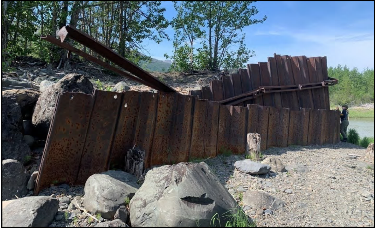
Figure 5.2-6. Feature 2 dam abutment on southern bank of the Eklutna Lake outlet showing damage from erosion. View to the west.
