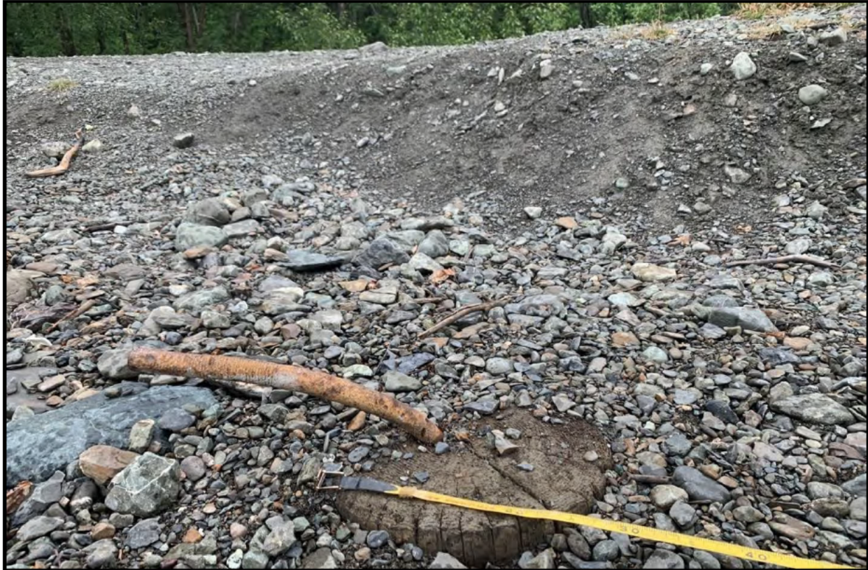
Figure 5.2-20. One of two log piers with threaded bolts. View to the northwest at the base of the Eklutna Lakeside Trail.
