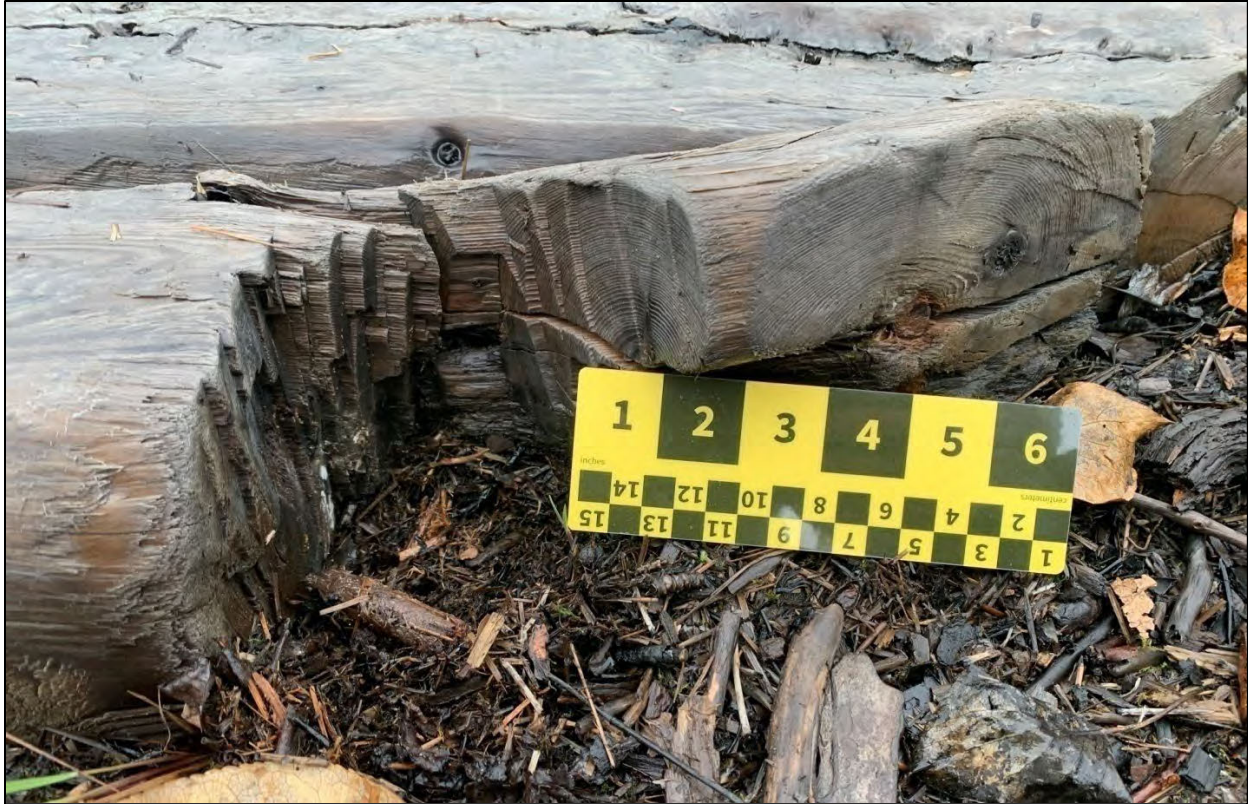
Figure 5.2-33. Detail of a hand-hewn corner notch of the Eklutna Alex Cabin. Ferrous staining of an iron spike can be seen in the log above the photographic scale.
