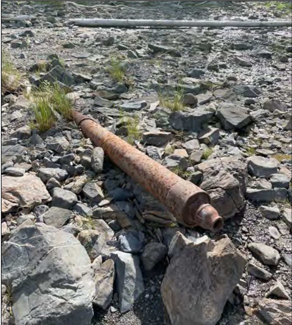
Figure 5.2-28. Metal pipe extending from the bank on the southwestern shore of Eklutna Lake.
