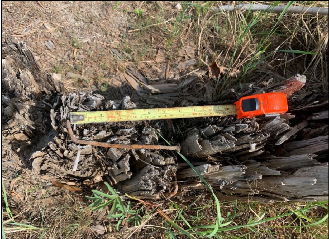
Figure 5.2-11. Detail of an iron spike and decayed vertical wood planks within Feature 3.
