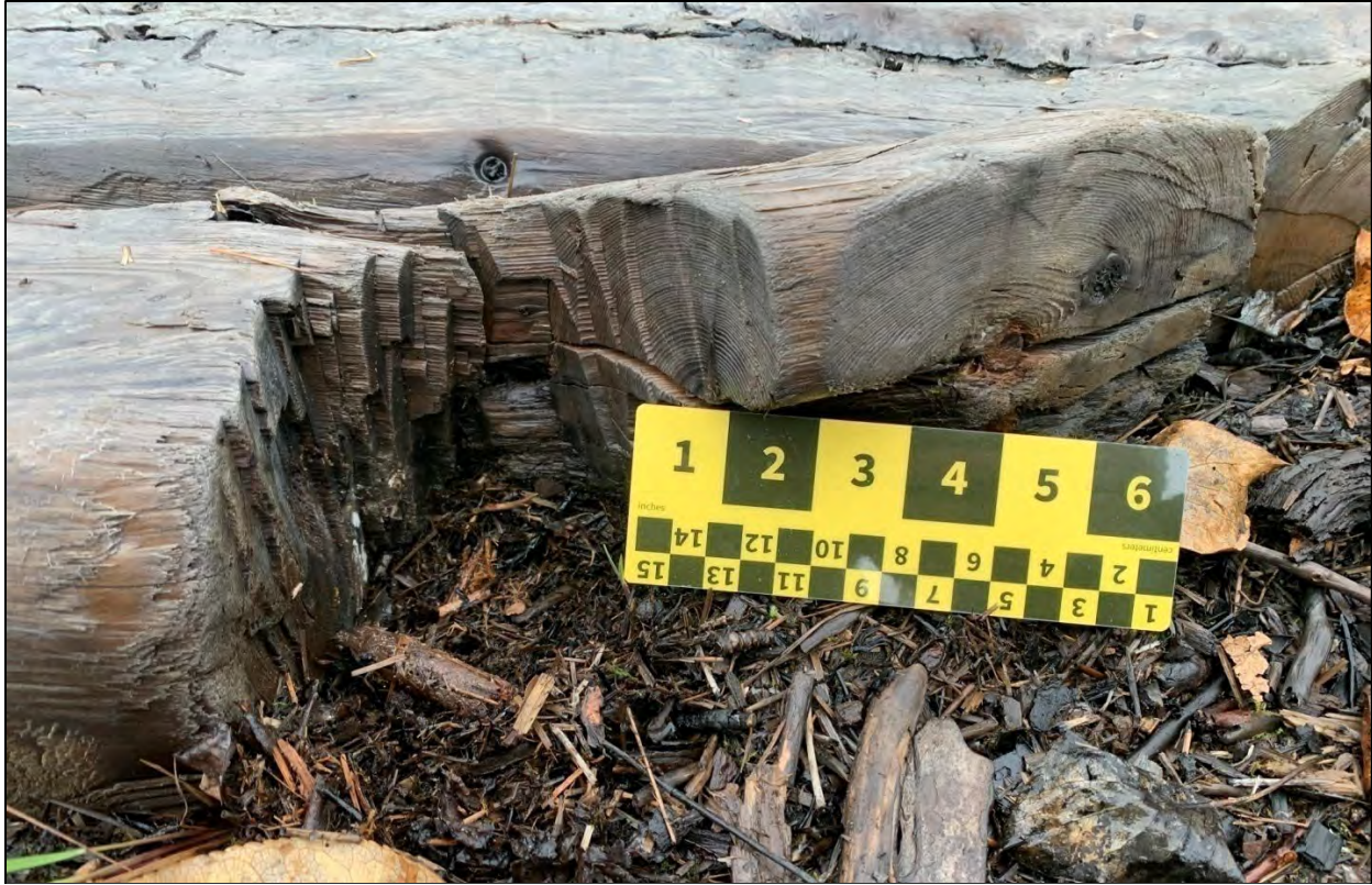
Figure 5.2-33. Detail of a hand-hewn corner notch of the Eklutna Alex Cabin. Ferrous staining of an iron spike can be seen in the log above the photographic scale.
