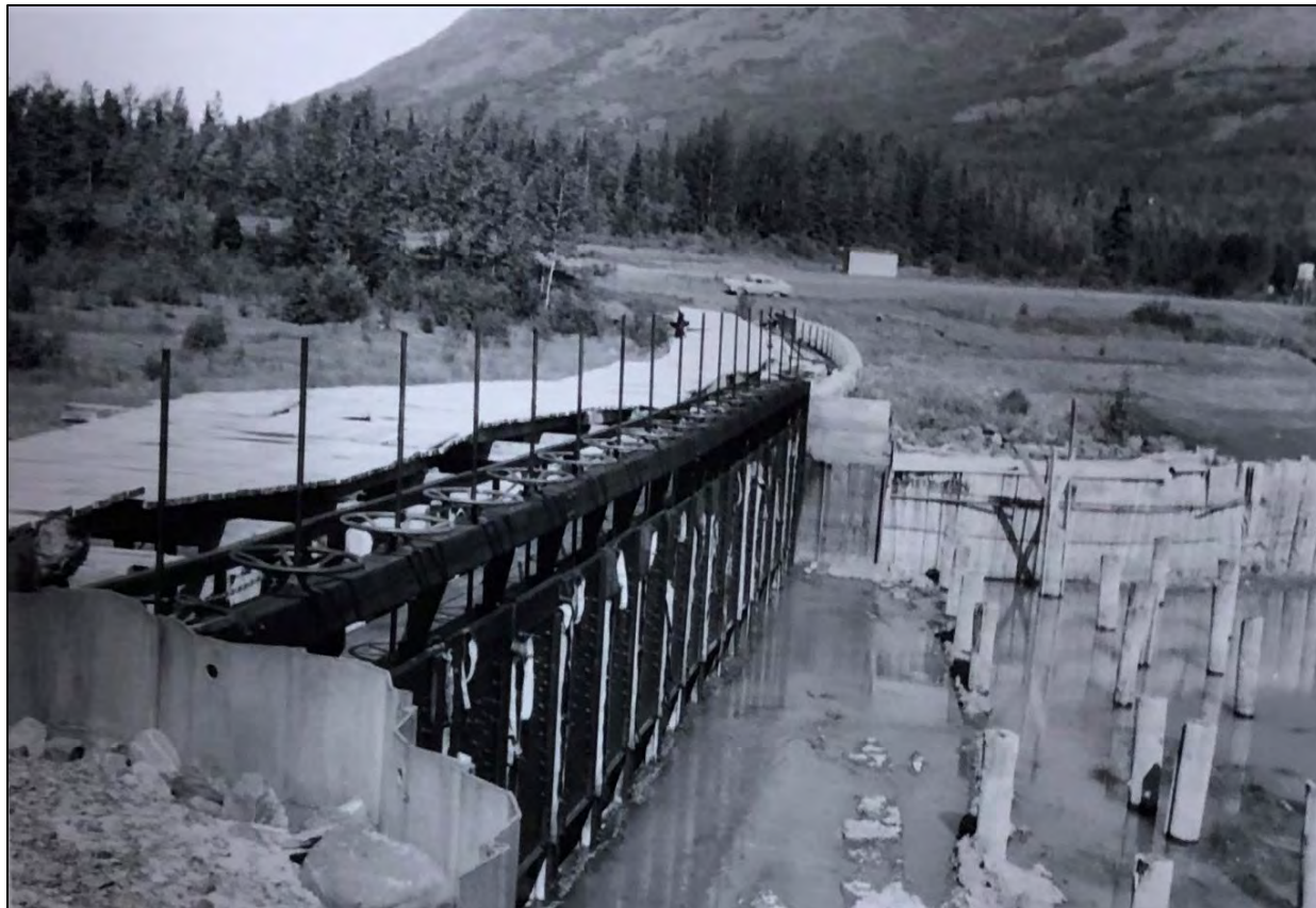
Figure 5.2-17. Photograph of the Eklutna Dam and Spillway following the 1964 Earthquake (USBR 1964:Plate 109). View to the northwest.
