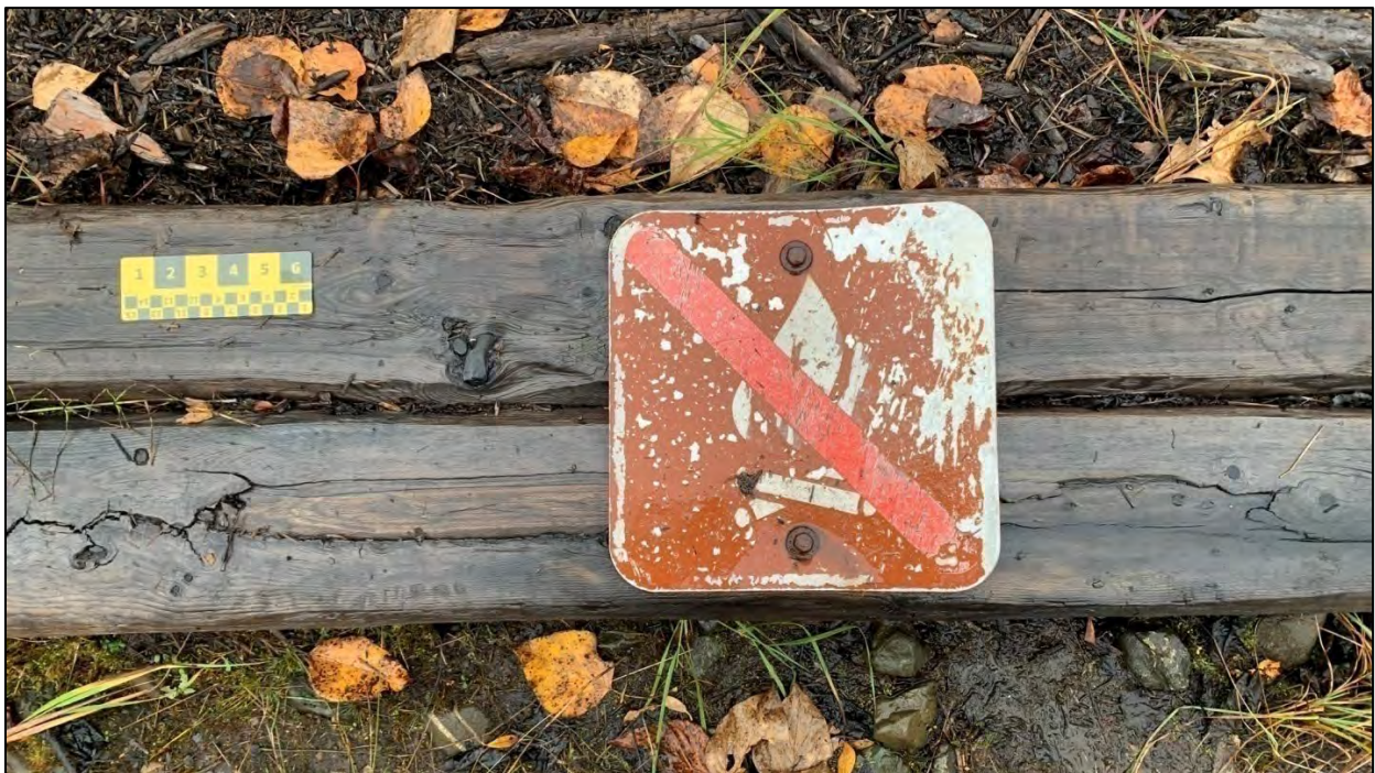
Figure 5.2-34. Weathered Chugach State Park sign bolted on what was once the upper gable wall of the Eklutna Alex Cabin.
