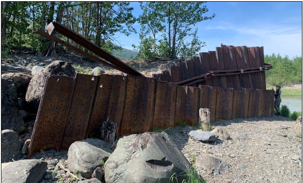
Figure 5.2-6. Feature 2 dam abutment on southern bank of the Eklutna Lake outlet showing damage from erosion. View to the west.
