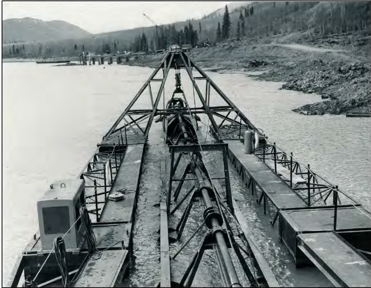
Figure 5.2-22. View of the temporary dock or wharf (background on shore) used during construction of the Eklutna intake tunnel.
