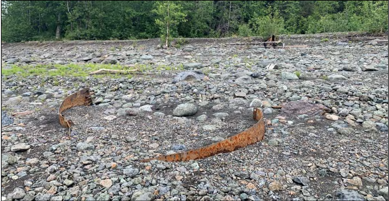
Figure 5.2-24. Steel repair band (foreground) and culvert along the Eklutna Lakeside Trail. View to the north.
